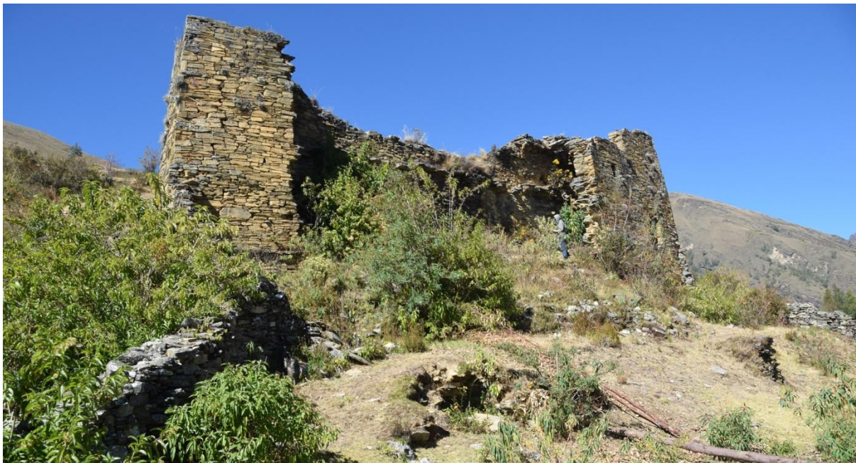
Interior face of the headwall, collapsed in the middle. Note the botanist at work.
