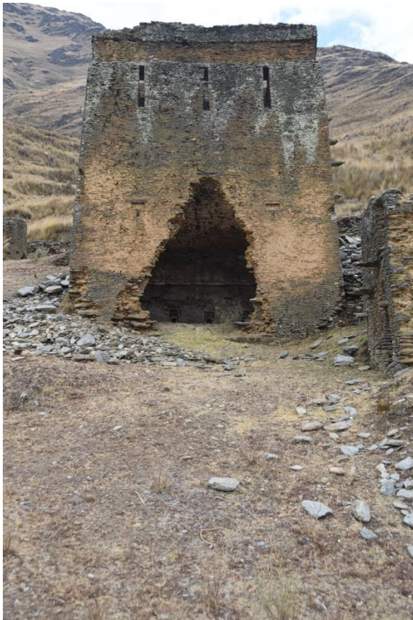
Mancopa: Fallen lintel over doorway
