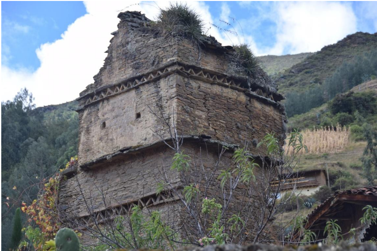
Upper half of the tower seen from below. Note zigzag decoration and cracks in the wall.
