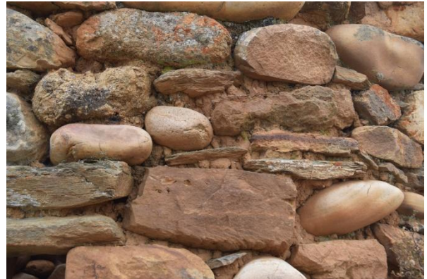
Gongui: Mortar washed out by the rain
