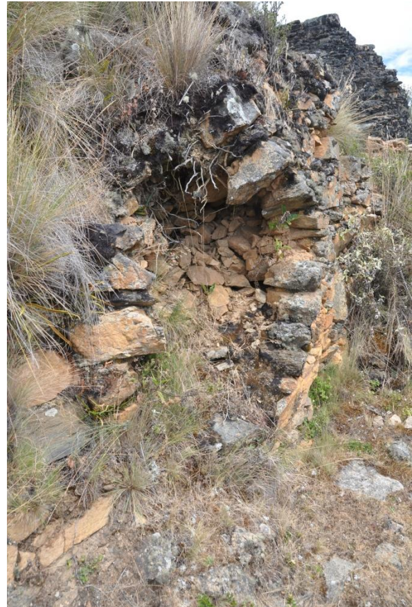
Pujin: Bulging wall
