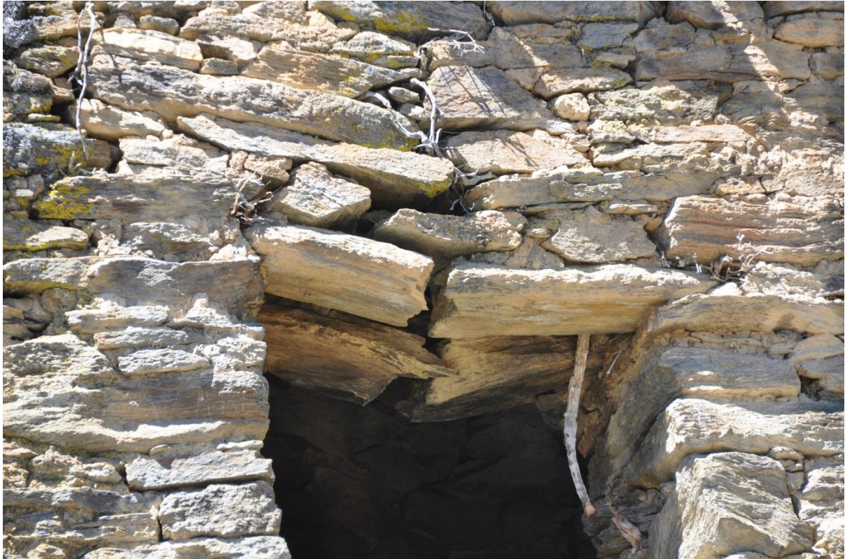
Broken lintel stones
