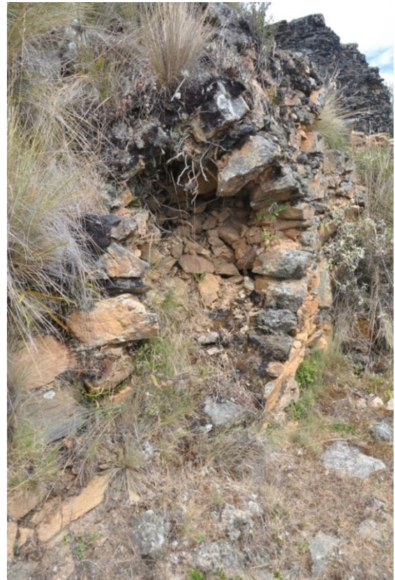
Wall waiting to collapse
