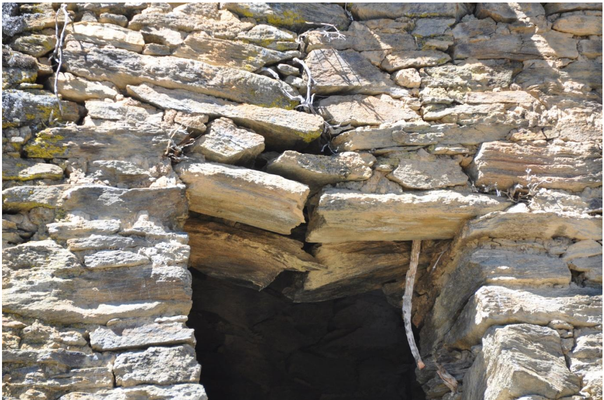
Ukru Rayan: Broken lintel stones are very common
