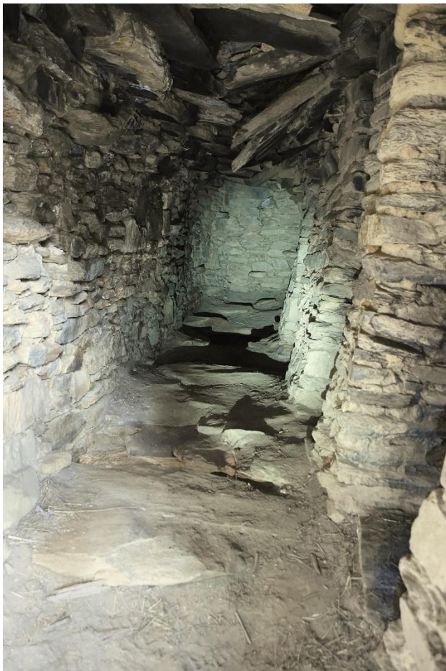
Gallery within the headwall. The walls and buttresses on the right really do lean that far over!
