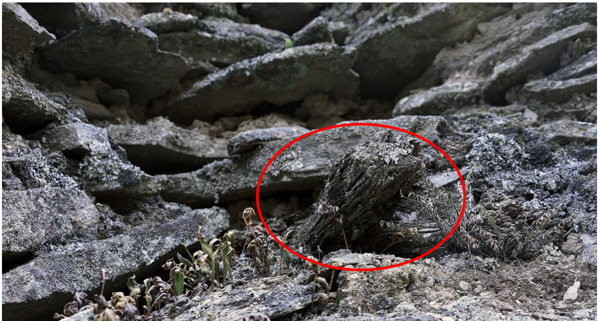
Beam end sticking through the roof, where the outer covering of the roof has broken away
